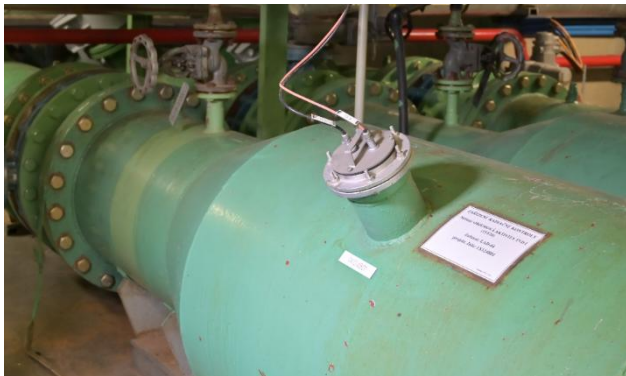
LAD-44 detector installed in the measurement sump within the process pipeline
