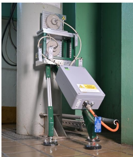
NGD-15 detector installed on the pipeline
